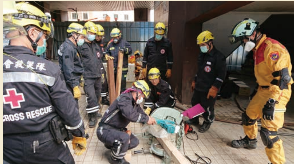
■臺北市舊南門市場-建物倒塌的破壞與支撐 Practice breaking and supporting a collapsed building in old Nanmen Market, Taipei City
